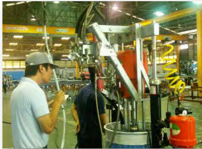
Glazing Pumps should be maintained regularly.
